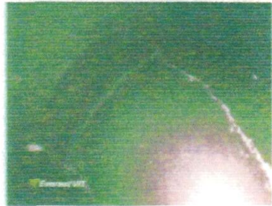
Strut and Start of Flow Conditioner
