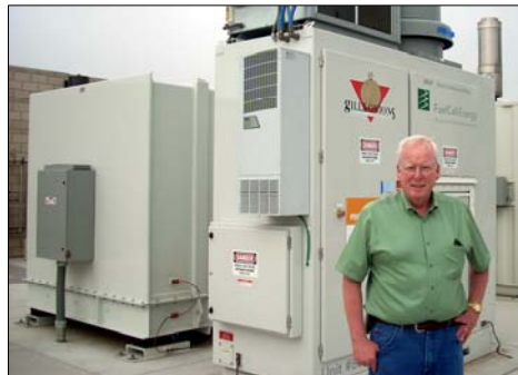
STEVE GILL IN FRONT OF ONE OF THE 300 KILOWATT FUEL CELLS AT THE OXNARD PLANT.
